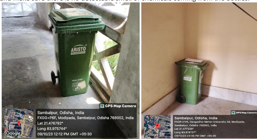
Dustbin installed at various places
