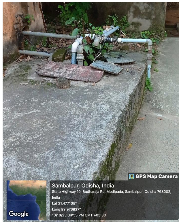
Pumping System at G.M. University
