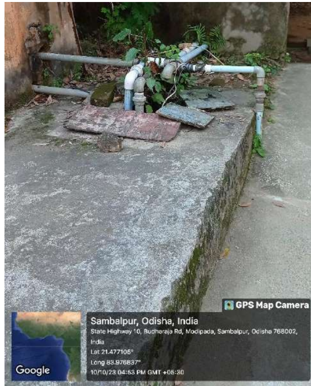
Pumping System at G.M. University
